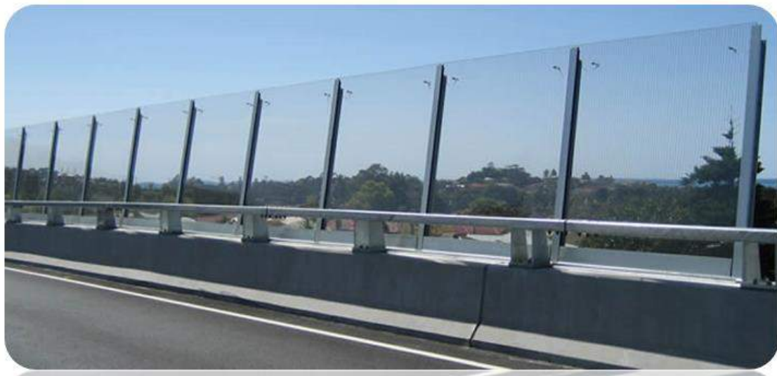
Figure 129: PLEXIGLASS sound stop noise barriers (Plastral 2017)
